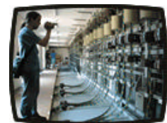
Recording the distributors of hydroelectric energy
